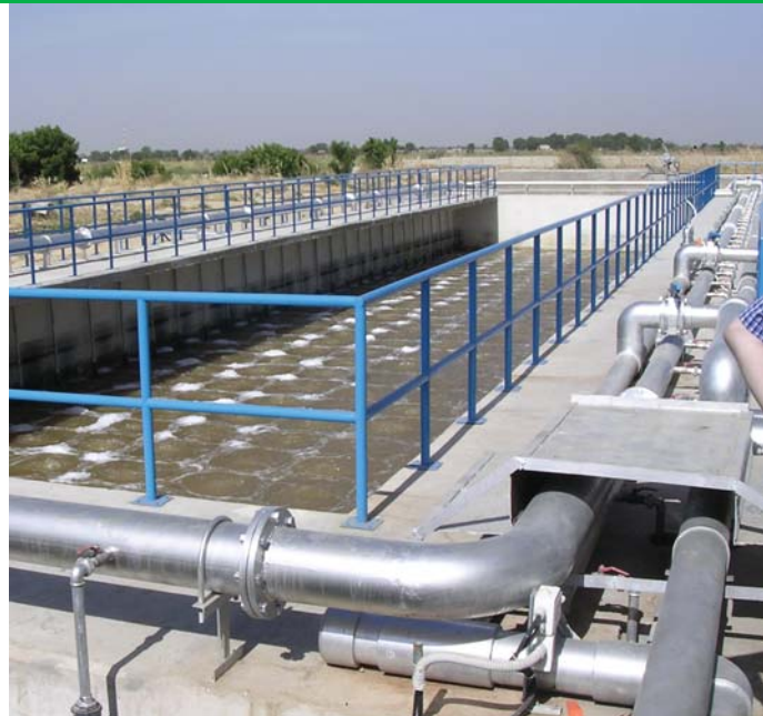
Wastewater treatment plant, Maidugury, Nigeria
