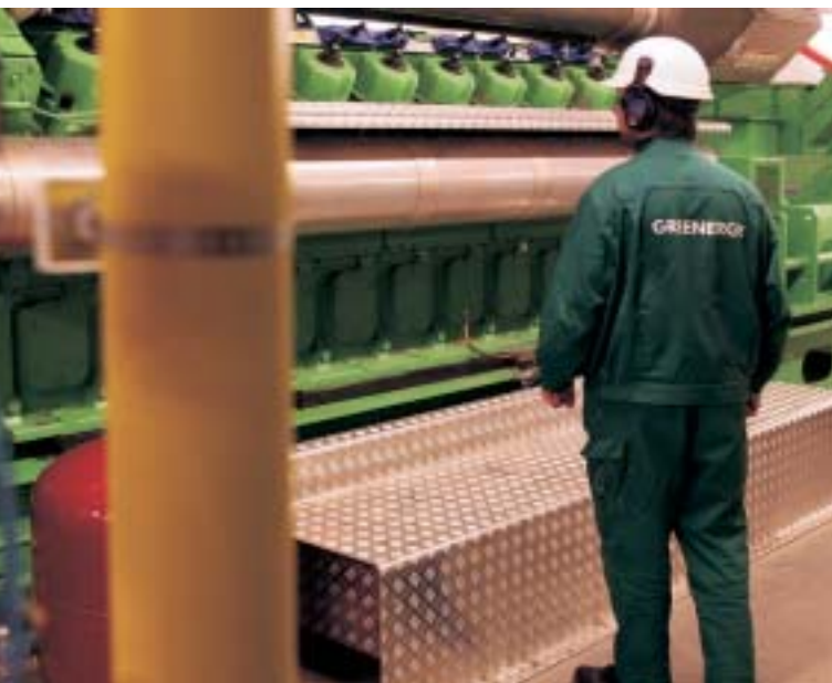
Coca-Cola HBC has identified a number of other potential sites to install the energy-efficient and emissions-saving power generation used at the Company's plant in Hungary.
