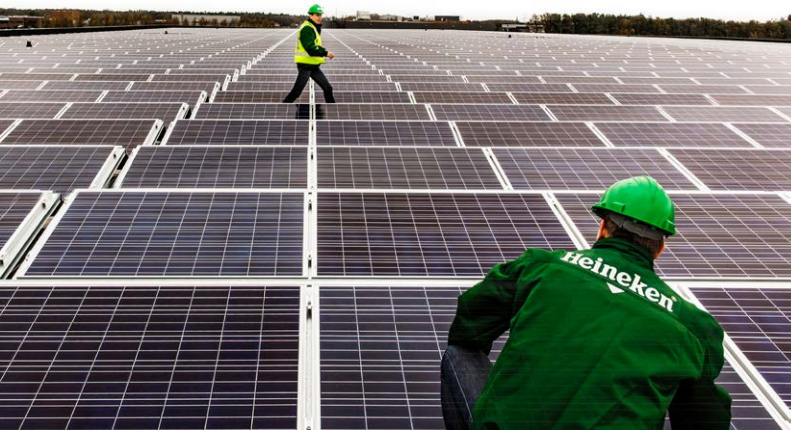
Final checks on new solar installations at eight HEINEKEN distribution centres in the Netherlands.
