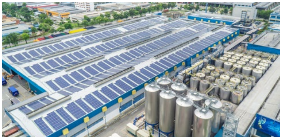
Solar installation on the rooftop of Tuas Brewery, Singapore.
